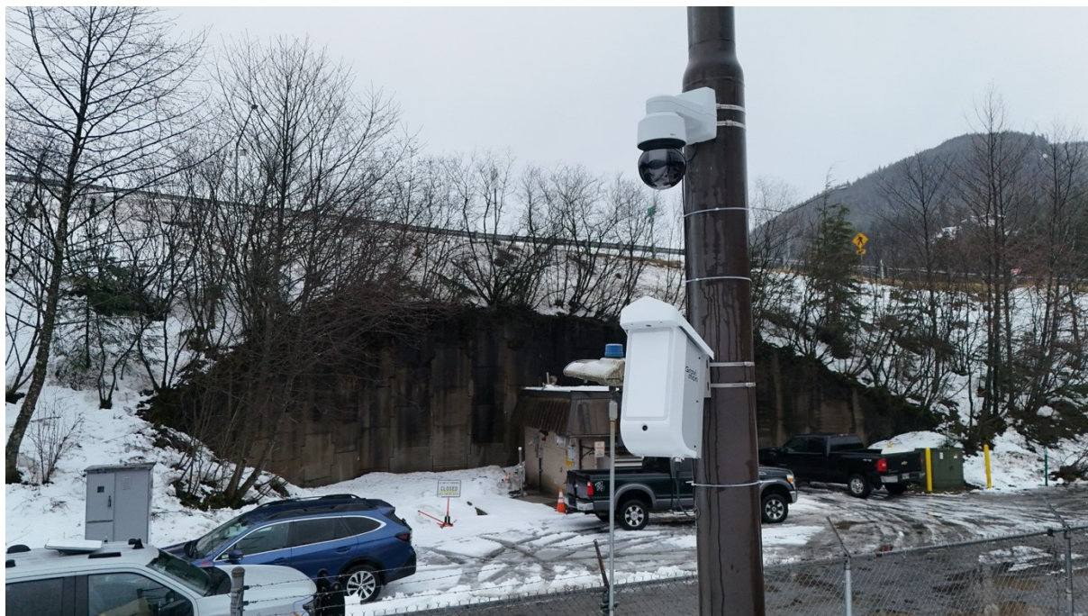
Figure 2: Gravimon avalanche radar and PTZ camera, installed at the AEL&P substation on Douglas Island, monitoring the Behrends path on Mount Juneau.
