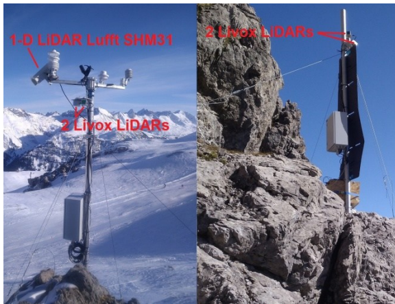
Figure 2: Installation at 2 different locations: Left: 2 Livox Avia LiDARs at a full automated meteorological and snow station, where power supply exists. Right: Energy self sufficient installation in an avalanche safe location in a rock wall.
