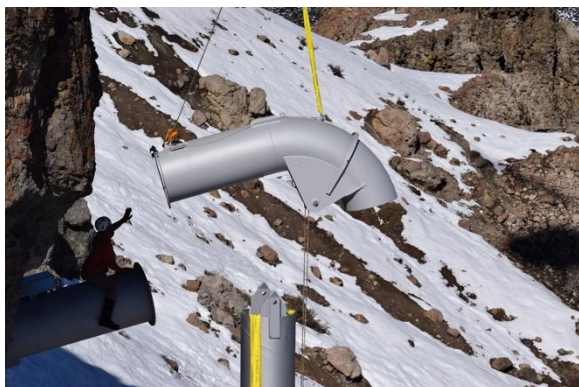
Figure 8: Gazex exploder replacement at Carson Spur, 2021.
