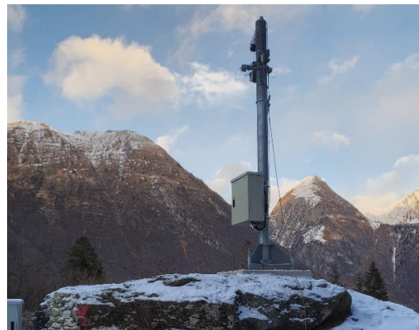
Figure 2: Installed avalanche radar system with the Toira slope in the background.
