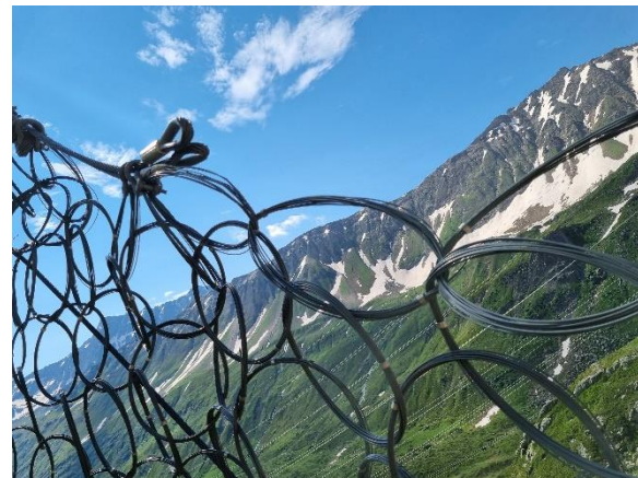
Fig. 18: Plastically deformed ring net close to top support rope on July 15, 2024, in Rosalba.
