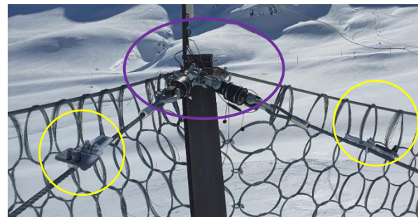
Fig. 8: Rockfall barrier at Chant Sura. Retaining ropes equipped with GUARDs (yellow) and "MicroStrains" (purple).
