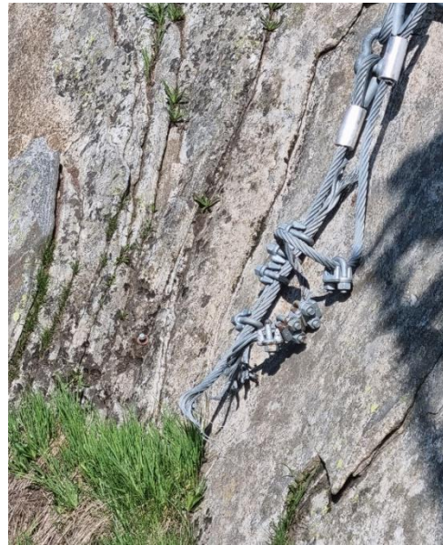
Fig. 17: Broken top support rope at rock connection on July 15, 2024, in Rosalba.
