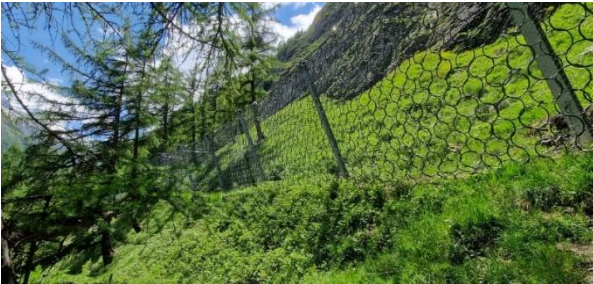
Fig. 7: Rockfall barrier at Arolla on June 15, 2023.
