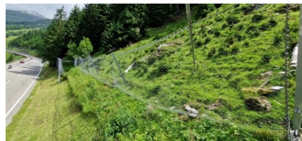
Fig. 5: Rockfall barrier at Felbertauern on July 4, 2023.
