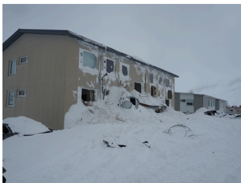
Figure 6: Apartment building below the Nesgöl avalanche path in Neskaupstaður hit by a snow avalanche on 27 March 2023. Photo: Ragnar H. Prastarson, 28 March 2023.
