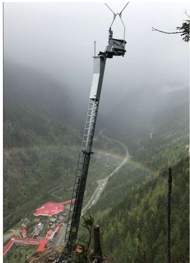
Figure 2: RACS installation at 3VG overlooking Trans-Canada Highway 1.
