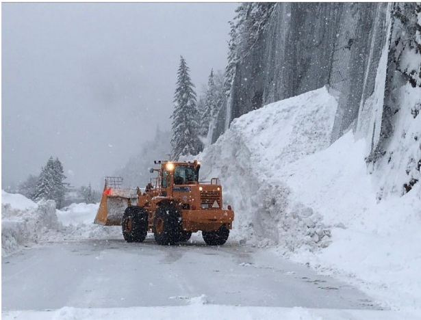
Figure 8: Avalanche debris removal at the rockfall drape net at Path 19.7.
