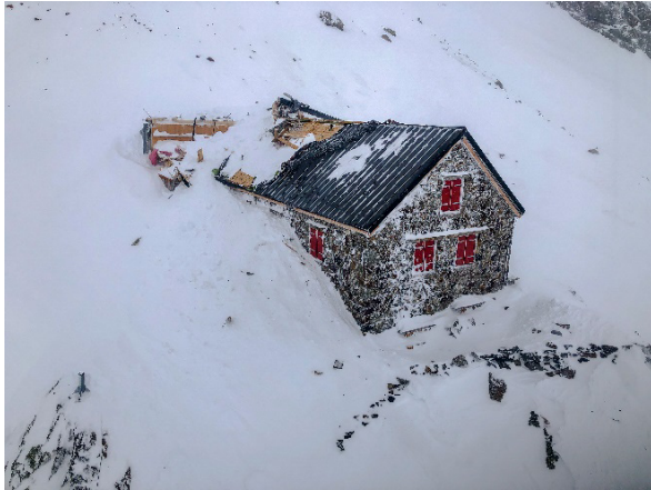
Fig. 4: The avalanche of 28 January 2021 destroyed the upper floor of the uphill extension of the Trift hut and tore away parts of the hut roof. Only little snow was deposited on the side of the hut. The snow plastering on the valley side indicates a powder component of the avalanche (photo SAC Bern).
