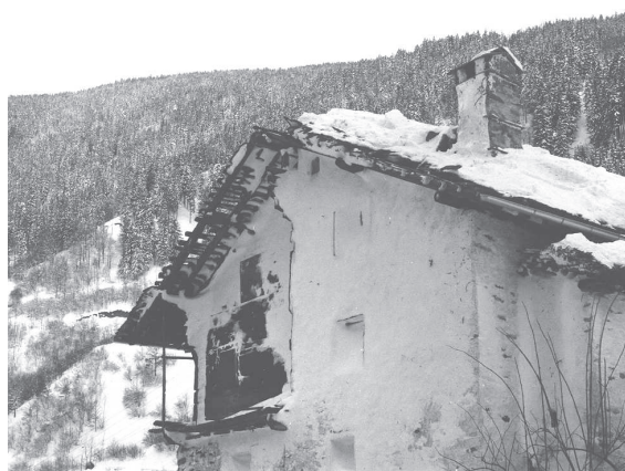
Figure 1: Signs of "air blast" impacts: top) snow deposits and damage caused by the 'skredvind' of the powder snow avalanche from Stortuva, Mosjøen, Norway, on 29.02.1996 (photo NGI); bottom) building damage caused by the Meira powder snow avalanche, Arviggio, Switzerland, on 12.01.1977 (photo Canton police, Grisons)
