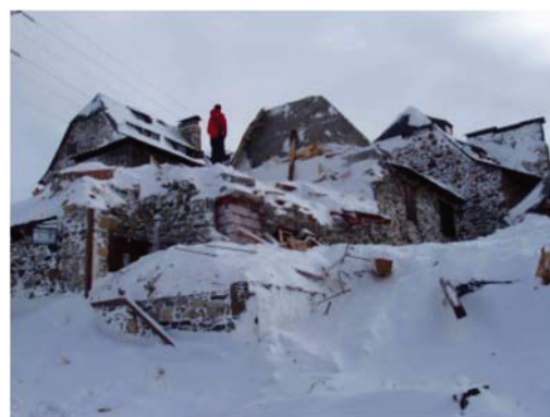
Figure 5: Structural damage to the front line of buildings in the avalanche area GAR203, January 31, 2003. Source: Avalanche Forecasting Survey of Aran.
