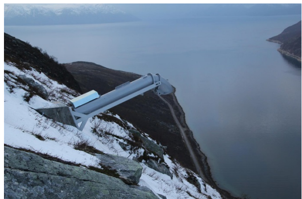
Fig. 3: Skillefjord Avalanche Area and road 883, Gazex exploder installed 2014. (Photo: Ole-André Helgaas)
