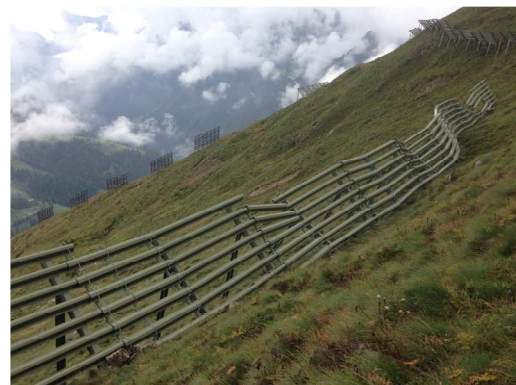
Fig. 9: example of damages in the crossbeams in the structure of snow bridges.
