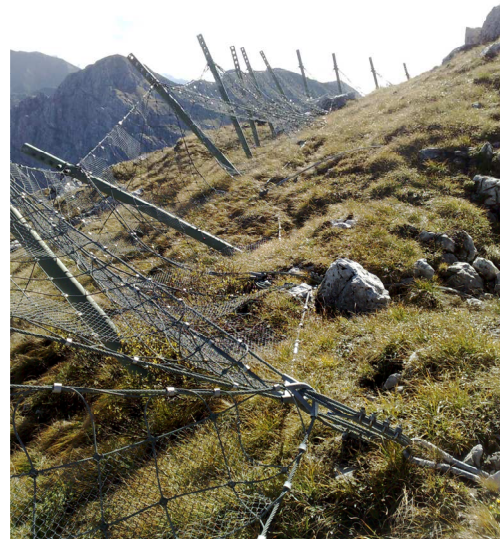
Fig. 8: example of damage in the structure of snow nets
