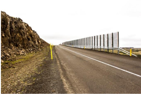
Fig. 7 The photo shows two sections of snow fences at the road side in summer time.
