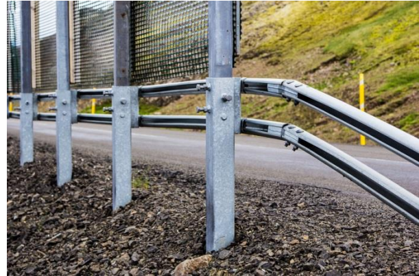
Fig. 9 A close up of one of the end posts. The guardrail end is bent down from the post into the ground.
