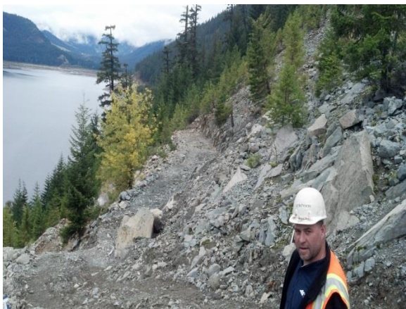
Figure 10. Initial grading of lower slide curve
