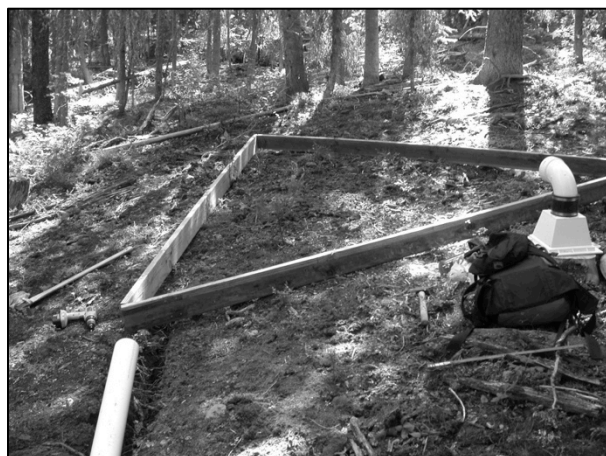
Fig. 3: Assembled frame for collection pan. Drain assembly, not yet installed and 4" elbow (upside down).
