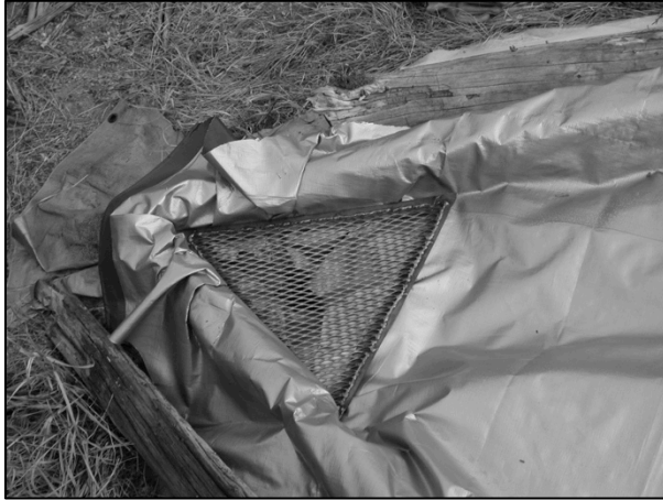
Figure 5. Lower apex of collection pan. A new tarp has just been added and small logs are placed along the sides of the collector to help hold the tarp in place until snowfall. Expanded metal screen keeps rodents and debris out of the drain assembly.
