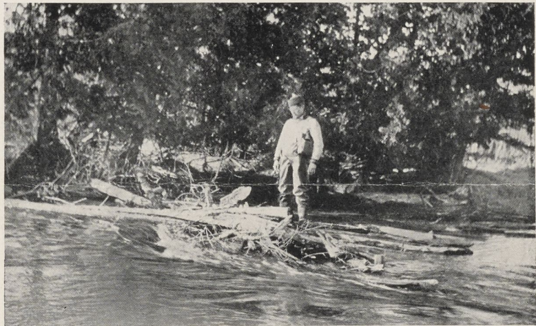
A current deflector installed in Pigeon River in the course of the stream improvement investigative work in Michigan. Note the great speeding up of the current and additional cover lodged on the barrier. Clarence Tarzwell, in charge of this work, is standing on a bar behind the barrier.
