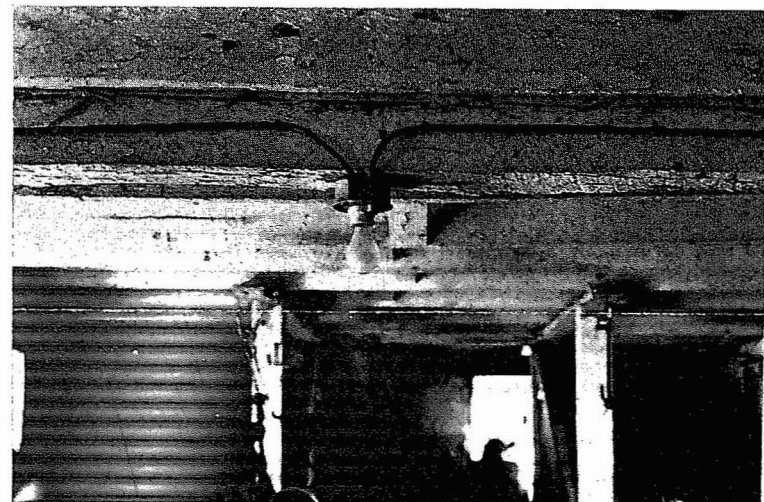
Figure 17. NON-METALLIC SHEATHED CABLE IN A DAIRY BARN.
