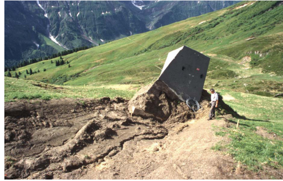
Figure 3: Foundation of pylon 7 of the 'Pleus' chairlift, Elm in spring 1999. Snow pressure has dislocated the anti-avalanche by some 8 m. The slope at the pylon is 28°, compared to other situations not really steep.
