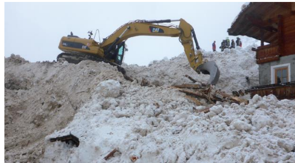
Fig. 17: farmhouse partially damaged, the 6 th Feb. 2014, by the avalanche at Pillhof - Moos in Passeier - [courtesy Bolzano Province, 2014].
