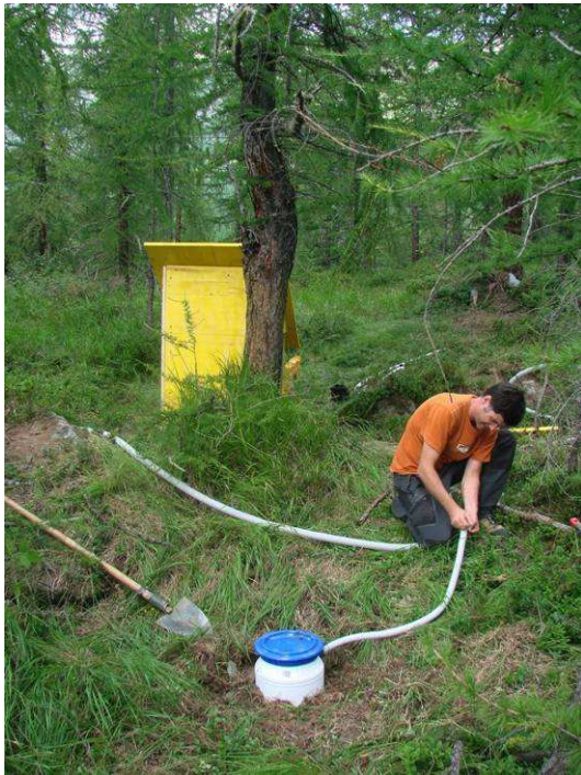
Figure 2. Array installation tasks in the forest (Summer 2012, Loc. Champdeleve – Valtourneche – AO, Italy). The infrasonic sensor is inside the blue box and the little yellow house contains the power and data transmission units (photo: N. Durand).
